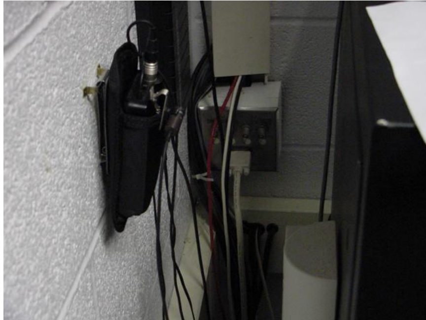
Undesired Smart Cart Input Box Coming Off the Wall
